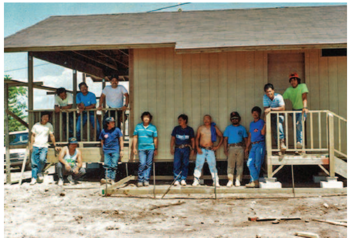
The Koga Crew building the Moloka'i house in 1992. From left to right: Top: Francisco, Noriel, Clay Below: Rolando, Benny, Rudy, Steve, Flor, Gil, Marciano, Nomer, Efren and Billy
