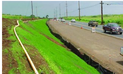
Slopes grassed and traffic lane prepared for a.c. pavement at South Leho Drive.
