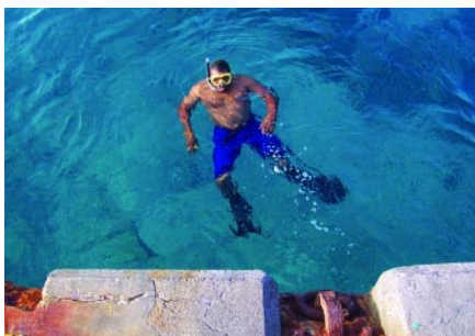
Swervin Irving "working" as he inspects the existing sheet pile corrosion.
