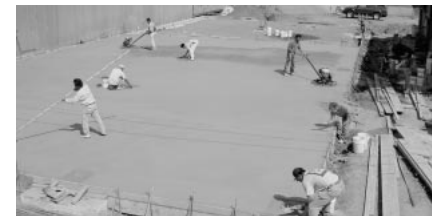
Work progresses on our new office building in the Sand Island Industrial Park
